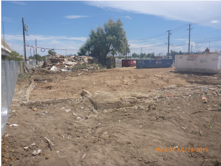
Photograph # 3 Alleged Violation # 1 View looking SE towards the footing of Building #2 (foreground) and Building #3 (background). The dumpsters are sitting where Building #1 once stood.
