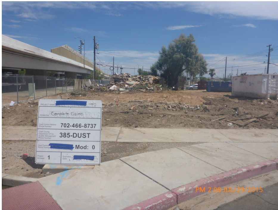
Photograph # 4 Alleged Violation # 1 View looking SE towards the footing of Building #2 (foreground) and Building #3 (background). The dumpsters are sitting where Building #1 once stood.
